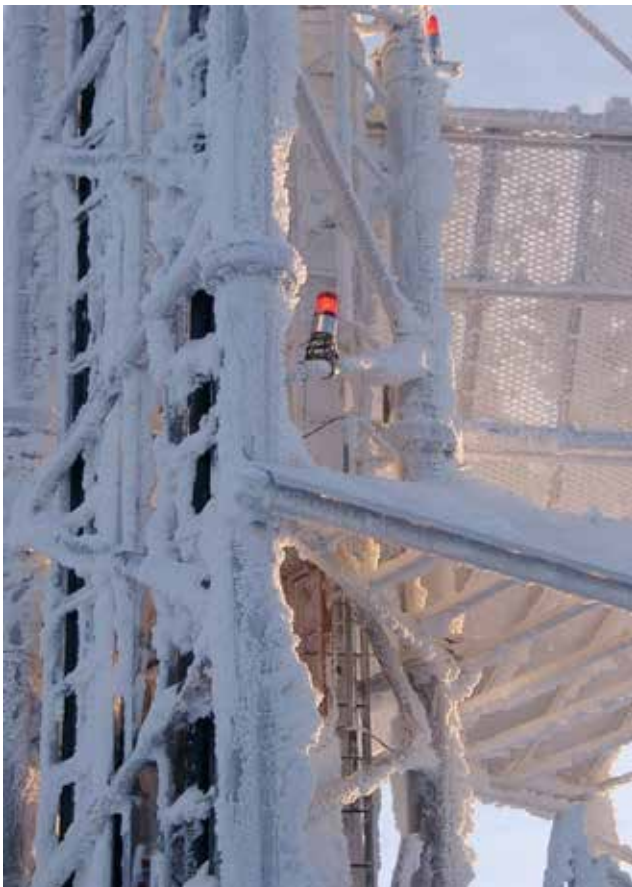
Installations have been carried out in Greenland, Svalbard and Kiruna.
